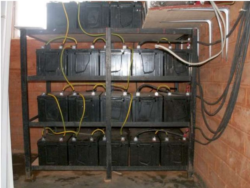
Figure OGP 9: A battery bank of 3600 Ah, currents reach levels of 45 A during charging
