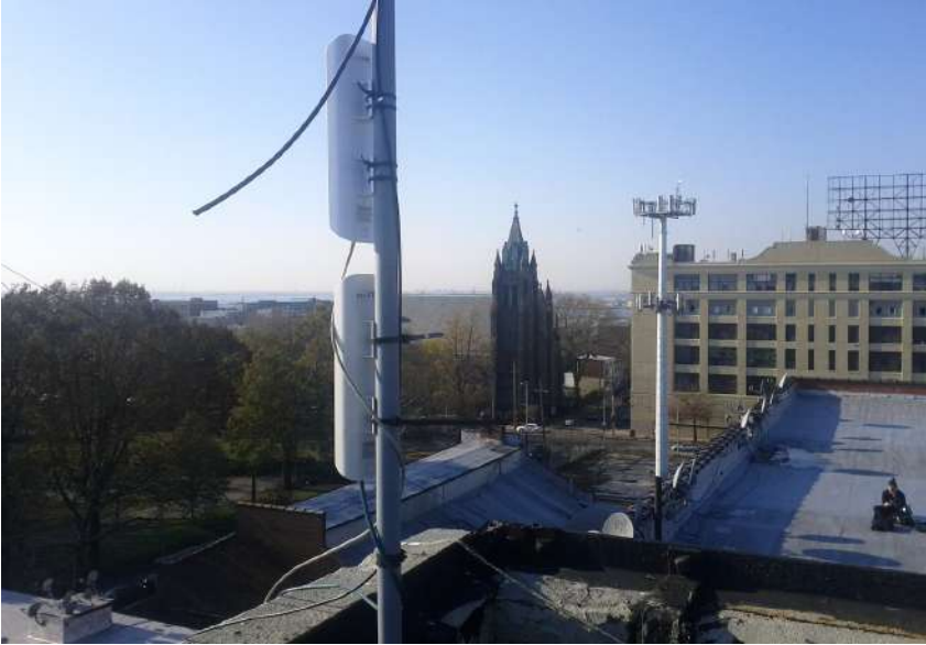
Figure CsOTI 14: Rooftop node installed after Superstorm Sandy.
