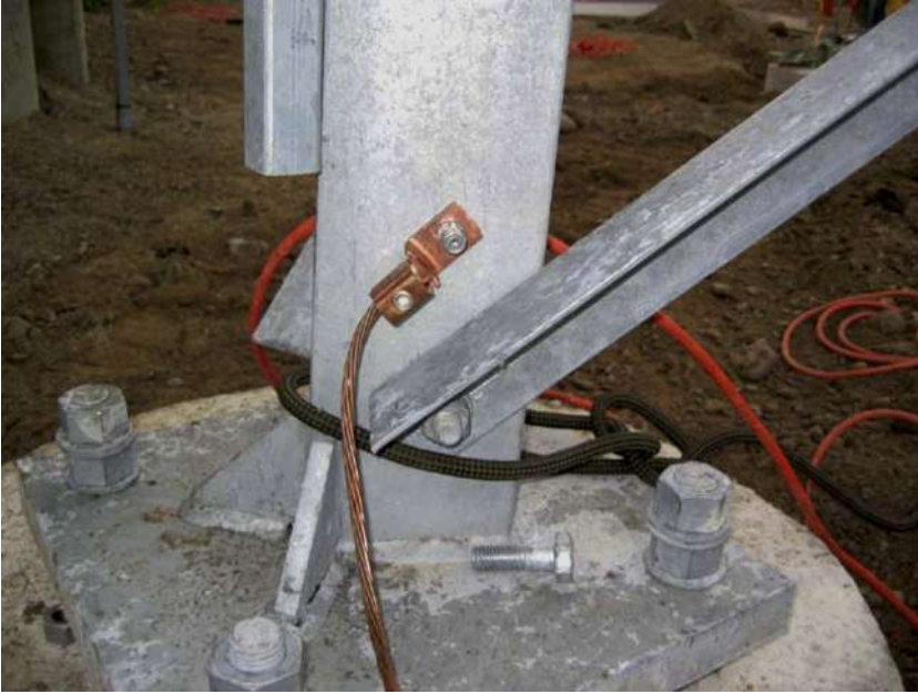
Figure HW 3: A tower with a heavy copper grounding wire.
